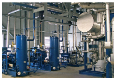
The Lutterworth site includes an ammonia and CO 2 plant
